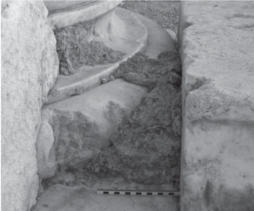
Fig. 32 Detail, cement fill between column base and statue base of the Tetra- style Court
