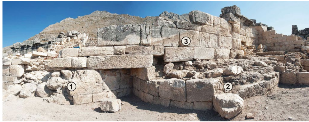
Fig. 6: Southern view of the southern walls of the Old Baths and southern caldarium (C2). Indicated are (1) the western apse, (2) central apse, and (3) the later wall constructed on top of the dismantled apsidal walls.
