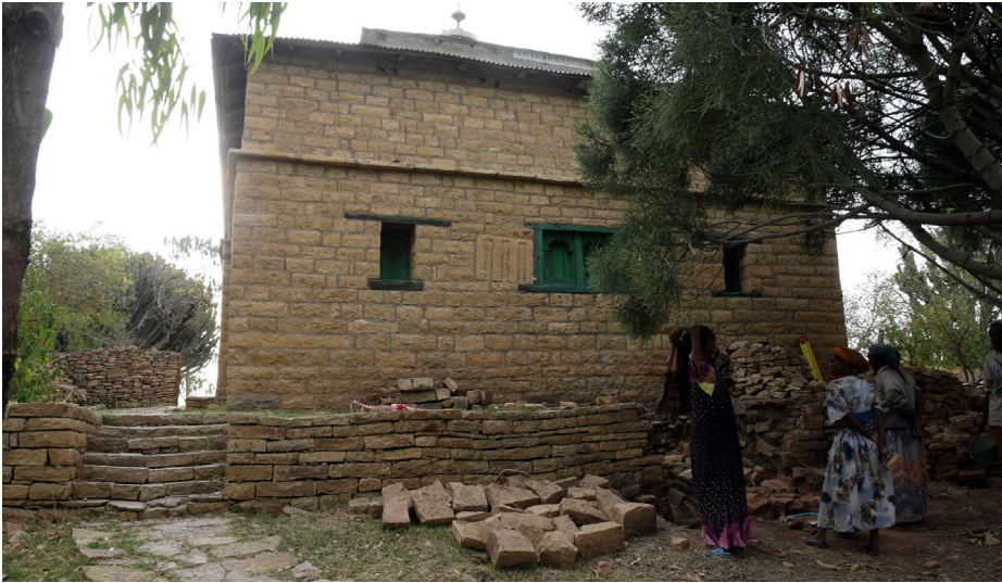
1 The church Abunä Gärima with cracked walls and spolia built within the walls (©DAI, photo: A. Lienig).
