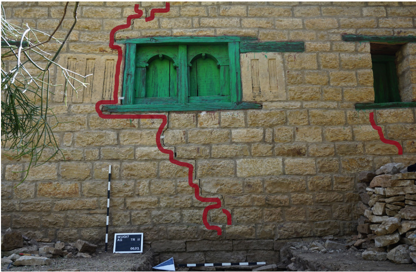
3 Western wall of the modern church of Abunä Gärima; largest fissures portrayed (©DAI, photo: S. Reichmuth).
