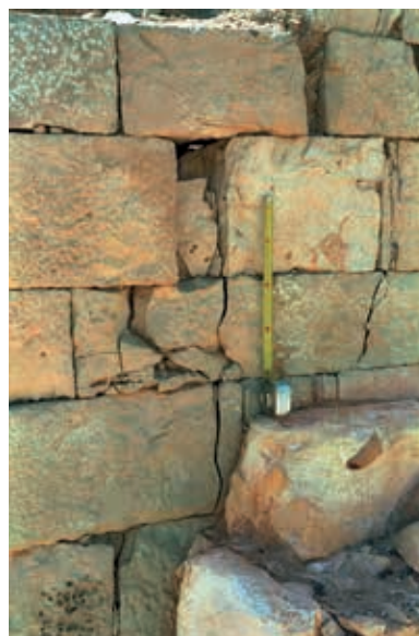
Fig. 17 Rehovot-ba-Negev, joints at the wall at the southern entrance into the Northern Church (field station 1) cut through three stones
