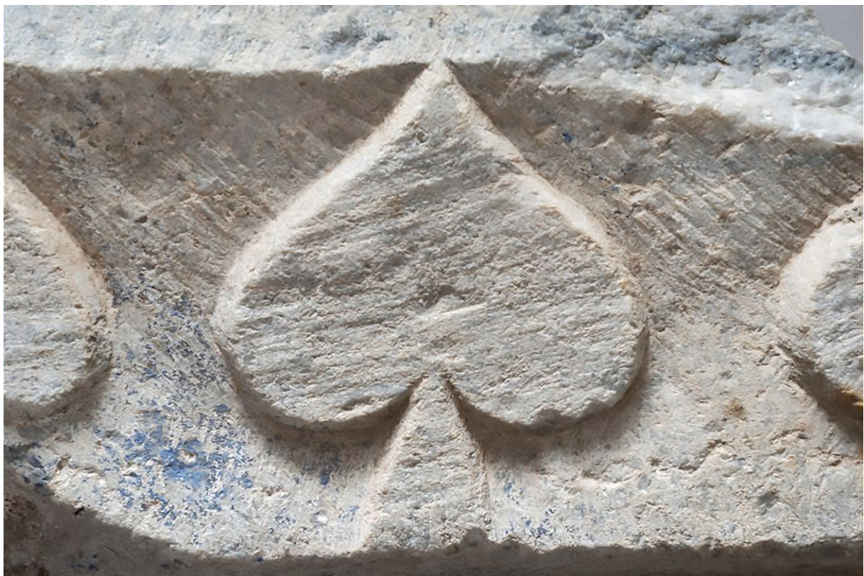
5 Istanbul, Küçükyalı. Detail of the frame of the Middle Byzantine church of the monastery of Satyros
