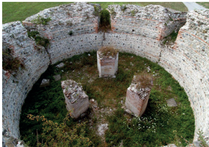
Fig. 6. Gramzigrad. Crack lines in the tower 19.
